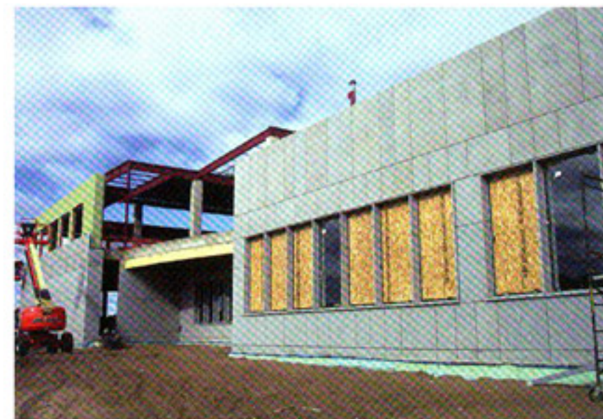
The new St. Cloud Public Library begins to take shape in downtown St. Cloud.
